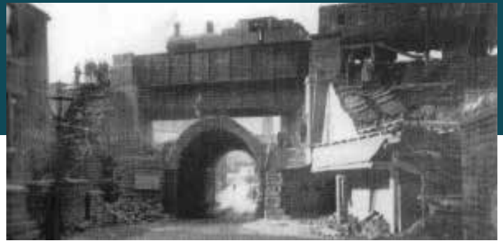
With complete disregard to safety, the new bridge functioning to the point where trains could pass over
