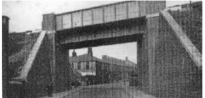
Seen from the Mount Street side following completion, now double deck-buses could pass through
